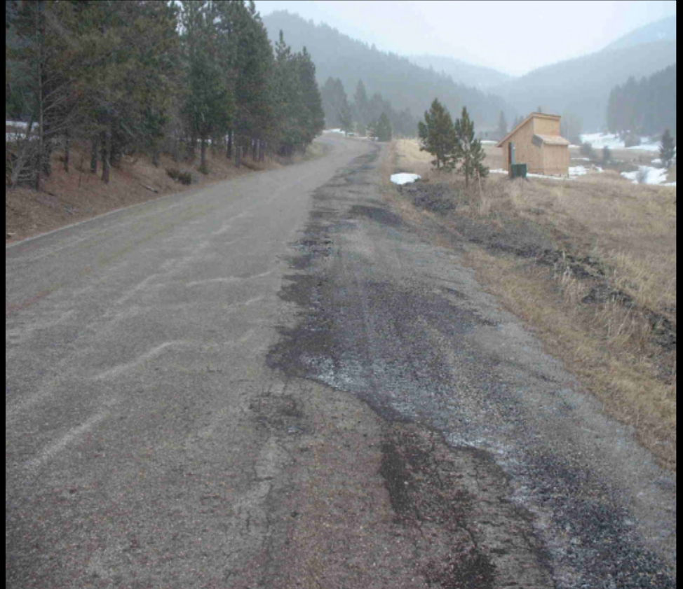
Road Department Grader/Patrol Damage circa.(2007)
